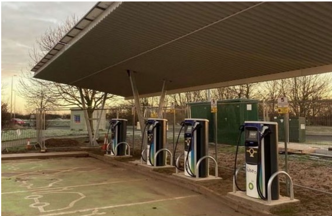
Figure 9: Gamston Community Hall Solar Electric Charging Hub
