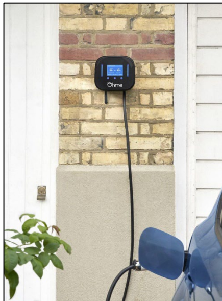
Figure 7: Example of new build EV charge point
